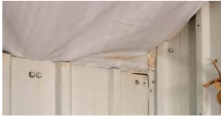
Fig. 14 Sharp edges in cladding [15]
