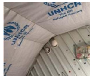
Fig. 17 Ventilation pipes closed [15]
